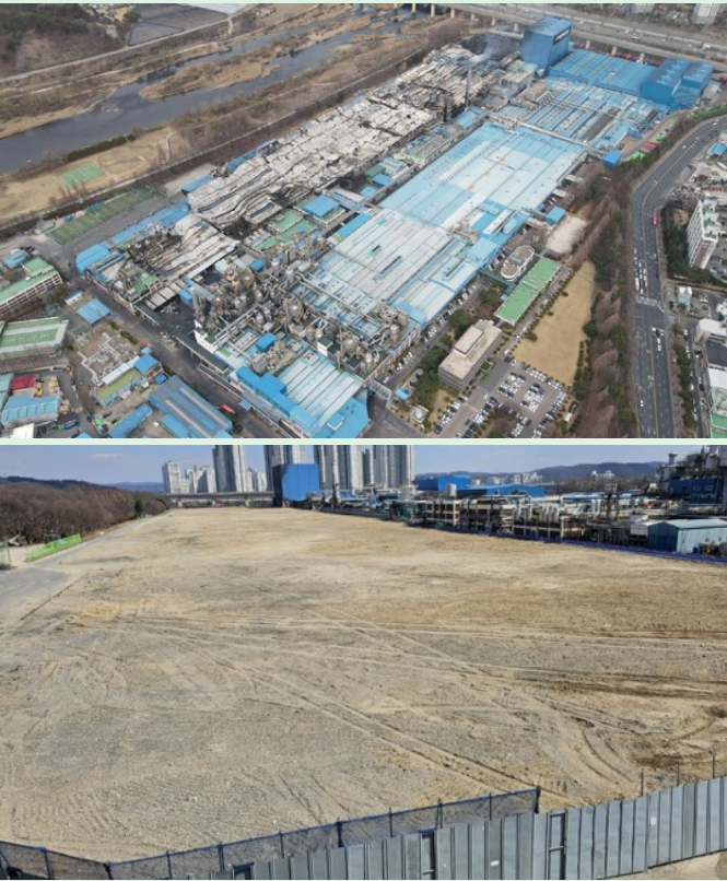
Daejeon Plant after fire (top) and after demolition (bottom)
